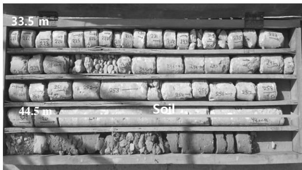
Figure 10. Concrete Core – Pile No. 1097 (Note the discontinuities and soft zones)
